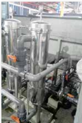
At our WWTP, a Filter Bag was added to remove balance residue from the next process, was amongst many of the on-going enhancements we have made as part of our IETS Improvement Plan
